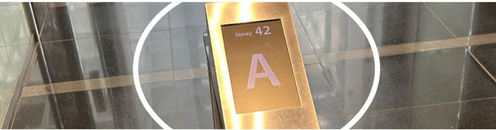
Turnstile screen confirming Storey 42, Lobby A.
